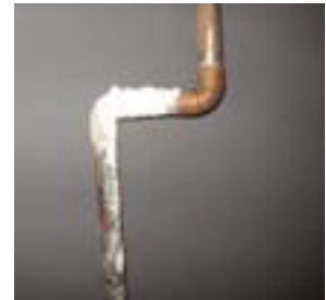
Hard scale build up on exterior of copper pipe in plumbing system.
