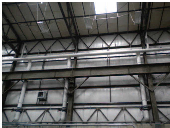
Interior Conveyance Piping Connecting Downspouts and Tanks
