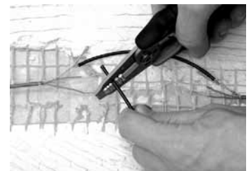
Step 4.13. Use the 16 AWG setting on the wire strippers to strip off exactly 1/2" of the insulation from both ends of the black jumper wires.
