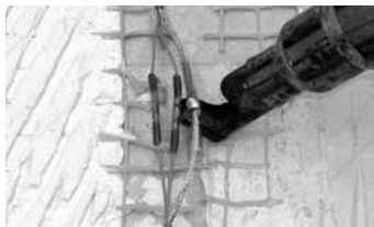
Step 3.17. Heat the tube to shrink it completely and cause the solder to flow into the twisted wires completely. When it cools, the connection should be secure.
