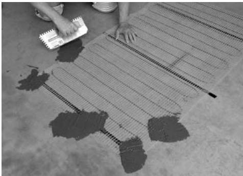
Trowel patches of quick-set to the corners and edges of the mat to secure it to the floor.
