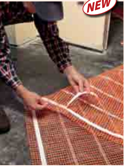
Roll out mat and secure to the floor using new adhesive strips.
