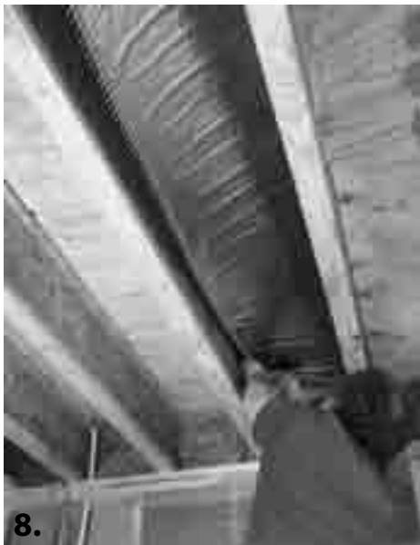
7. Continue stapling the mat mesh at 2" below the sub-floor, every 4" to 6". Then remove the nail at the end that held it up.
