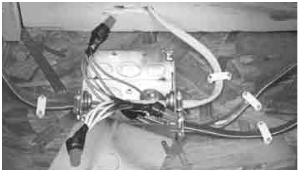
Junction box with multiple sets of mat lead wires, connected in parallel, and connected to the SunStat control above.
